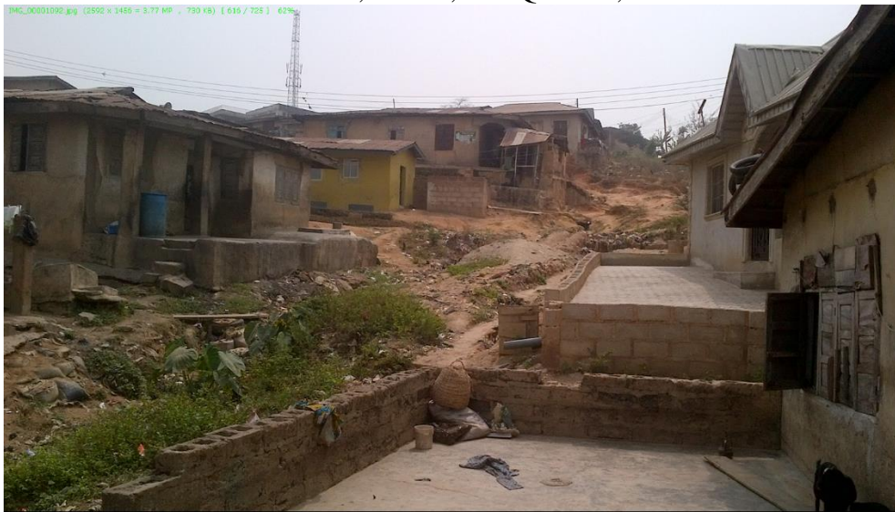
Plate 1.0: Failed Service Road, Balaro, Old Quarters, Ibadan
